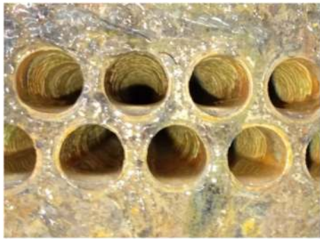
Scaling deposit in a condenser
