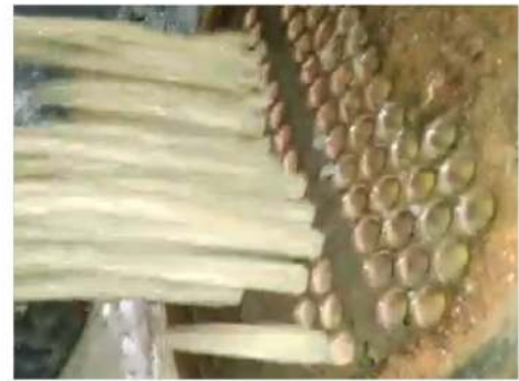
When the lid was opened after 60 days all the existing scale was removed and was drained away with water without use of chemicals or efforts.
